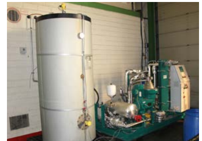
Part of the heating system for used cooking oil
